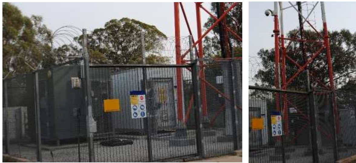
QBE4 - Transmission tower positioned at point QBE4. The facility is accessed via a narrow bush track and is fenced off with razor wire for security purposes.
