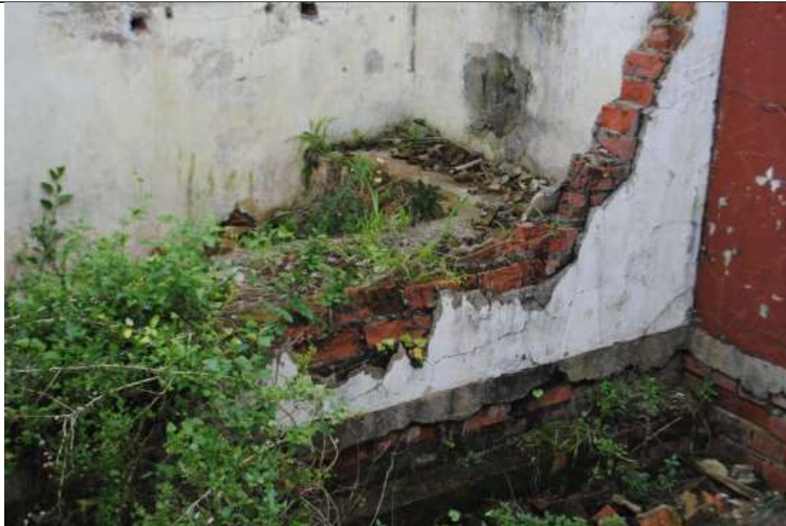
QBE3 – The remaining walls of outbuildings walls are damaged, with exposed brickwork and vegetation growing in the walls.
