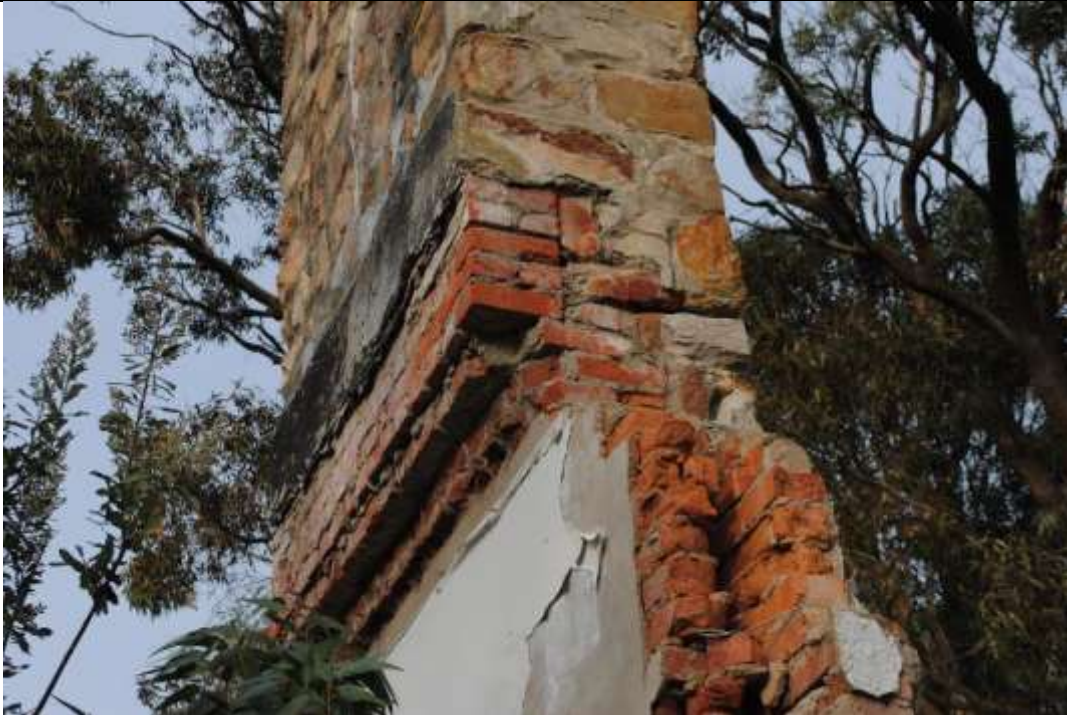
QBE3 – The chimney is partially intact and built of bricks with some stone masonry. The bricks have become brittle, while the stonework has remained in a reasonable condition.
