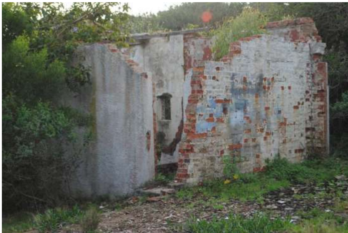
QBE3 – There are no doors, windows, roofs or fittings left and the remaining walls appear to have started crumbling in places.
