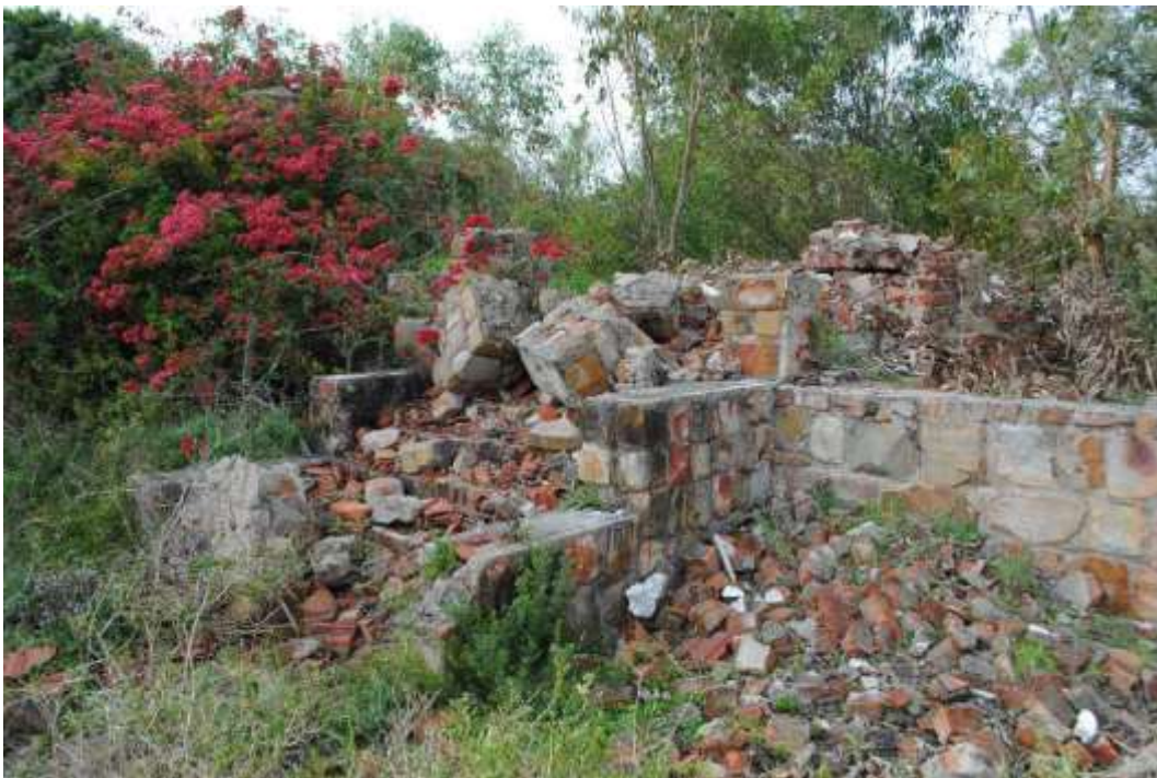
QBE3 - Remnants of the staircase of what would have been considered the front door to the building. Note the excessive building rubble as a result of the demolition and dismantling of the building.
