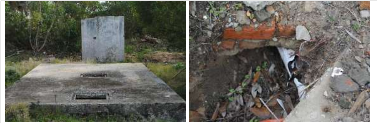
QBE3 – The existing building service infrastructure is in poor condition.
