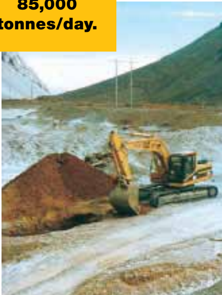
Test pit in the Pelambres valley for the study of the future waste dumps location
